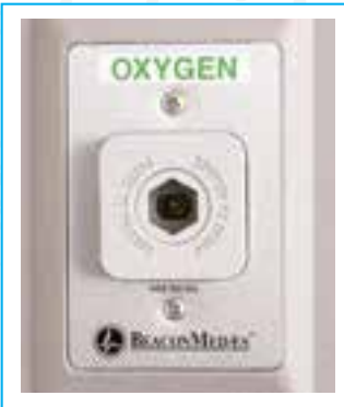
Gas Outlets Valves & Pipeline
